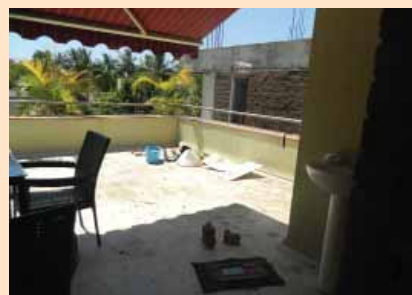
Completed terrace with water pipes below tiling and high albedo paint above
