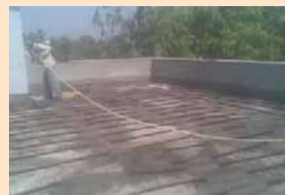
Laying out the coil of pipes above RCC slab with screed below tiling at the time of construction of terrace
